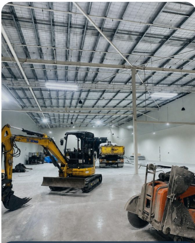
Inground Hydraulic Services
